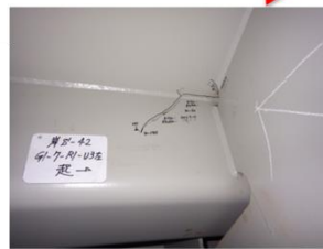
鋼床版のき裂
