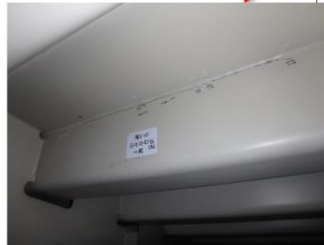
鋼床版のき裂
